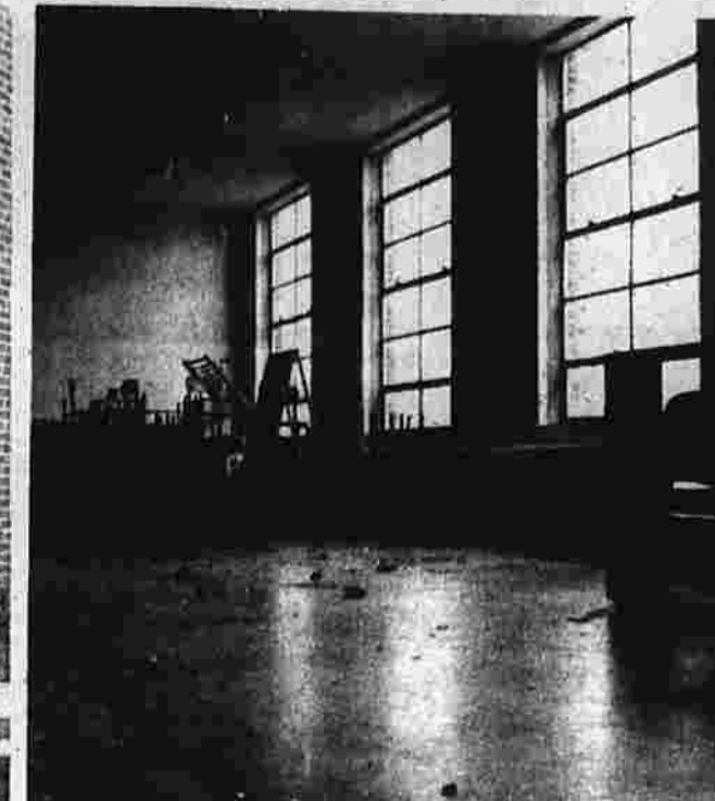
This was the damage done over the weekend by a group of vandals at Buckley School, Vernon St. Approximately 35 windows were broken in an apparent rock-throwing spree at the school. Ted Fairbanks, superintendent of school grounds and maintenance said that the damage done to the windows would cost the town over $1,000 to repair. (Herald photos by Knapp)
